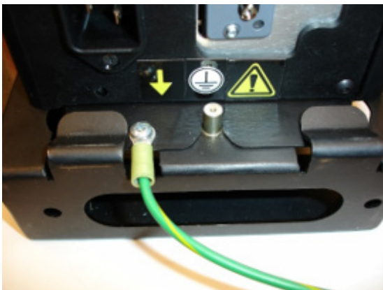
Figure 1 — Redundant Earth Ground Attachment
